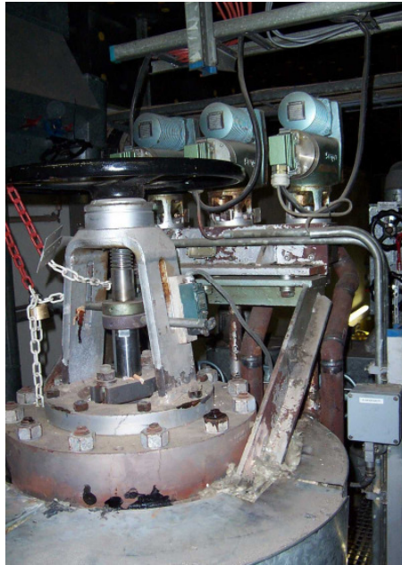
Original condition of the main valve with conventional control valves
